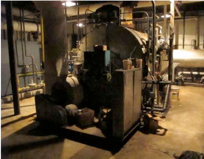
Single zone boiler
